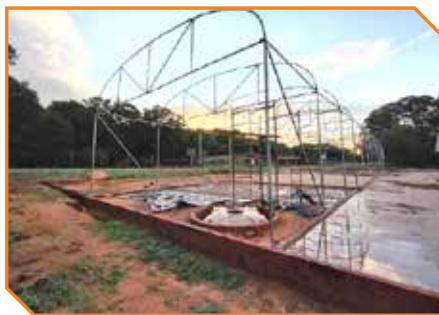
Floor of the structure after a heavy rainstorm
