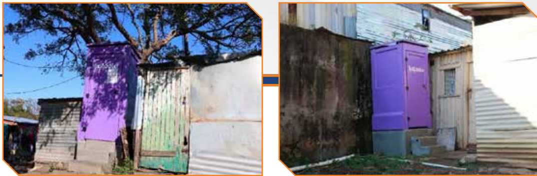
Figure 23: Kaloola toilet installations in an informal settlement in Durban
