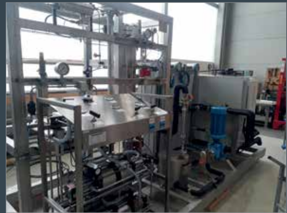
Figure 12: The constructed continuous supercritical fluid extraction plant
