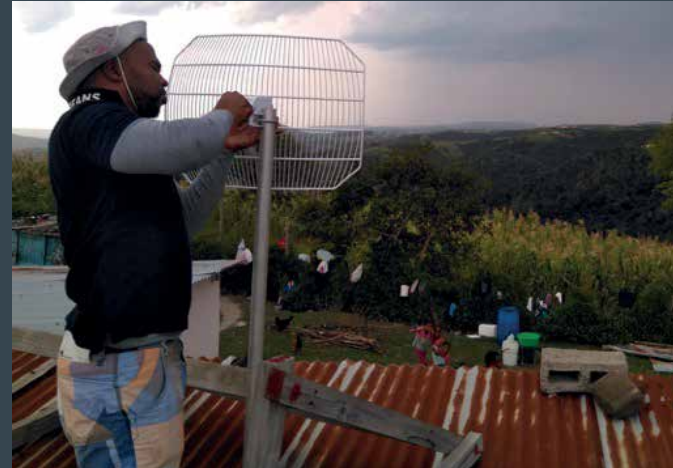
Figure 27: A technician from the community conducting maintenance of the Zenzeleni “do it ourselves” Connectivity Initiative equipment
